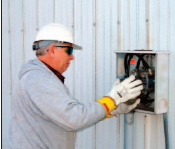
Conversion of current meters to AMR units will occur beginning in late May or early June.
